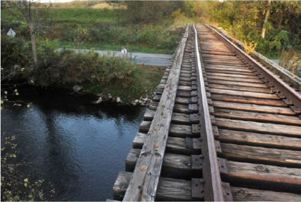
Hendersonville-Pisgah Forest unused rail line, as it crosses on a trestle over the Davidson River Road and the Davidson River northeast of Brevard, just upstream from the Davidson River-French Broad River confluence.
